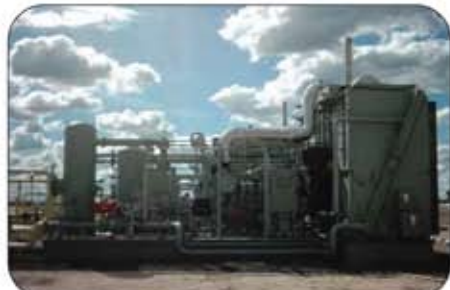
Less than 30 percent of the oil and gas industry's US field sites are remotely monitored. However, installing these capabilities in just one piece of field equipment, such as a gas compressor like this one, can yield significant ROI and increases in operational productivity and efficiency.
