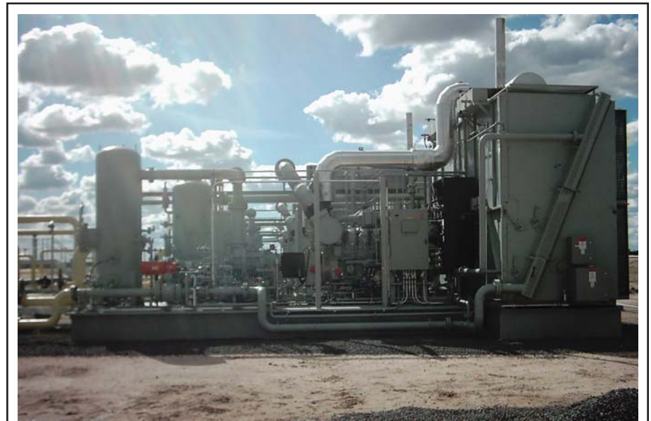
A "dispatch mode" of automated operations allows companies to constantly monitor compressors and other equipment in real time from a central control room. Using the data trending capabilities of a SCADA system, control room operators can dispatch field technicians as soon as a problem is detected. Leveraging remote monitoring to proactively address field problems and avoid shutdowns saves hours of production time and significant costs, while also providing HS&E benefits.
